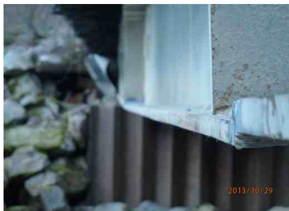
Figure 1-15: Offset weld in upstream girder.
