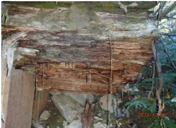
Figure 1-26: Left abutment- ballast wall - rotten logs.
