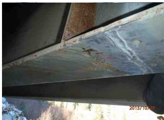
Figure 1-13: Typical previously repaired butt weld.
