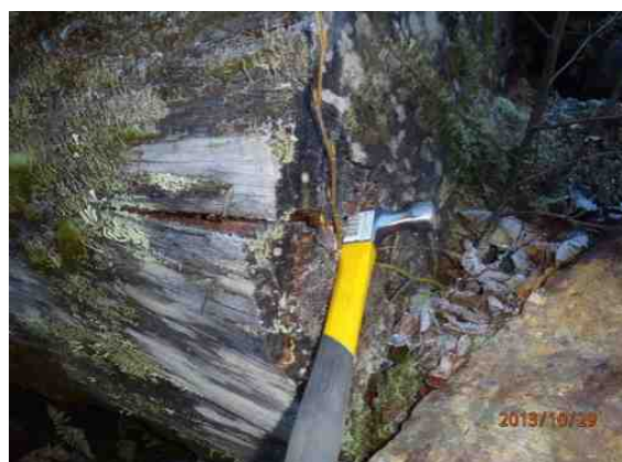
Figure 1-22: Right abutment - rotten ballast wall log.
