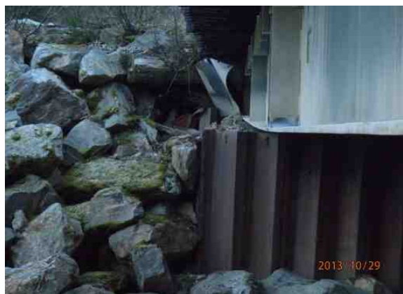
Figure 1-11: Sag in upstream girder.
